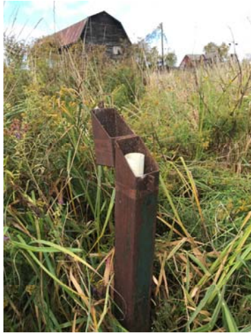
Photo 13: monitoring well OW17 (October 2020)
