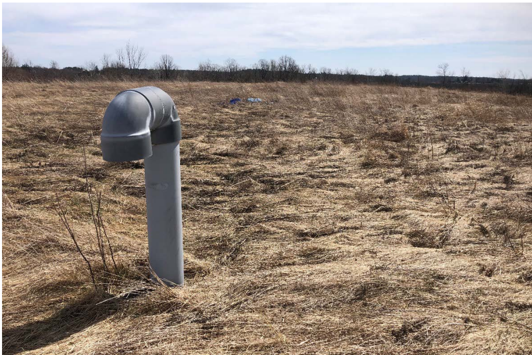
Photo 6: View of methane vent looking south.
