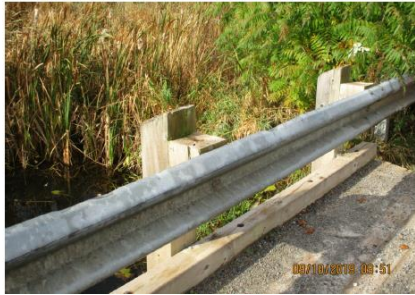
Steel Flex Beam Condition; Evidence of Localized Dent
