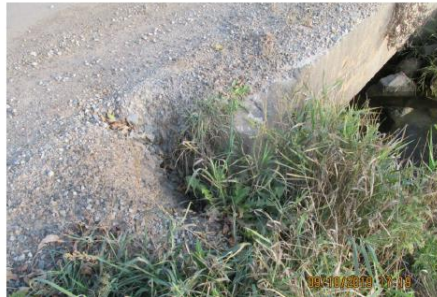
NW Embankment; Evidence of Severe Erosion
