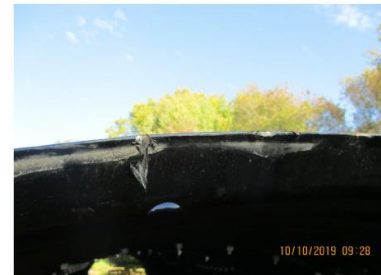
Culvert Barrel Polymeric Coating Condition; Evidence of Minor Scratch
