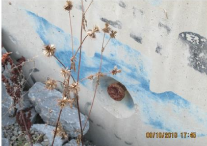
Culvert Anchor Bolts; Evidence of Minor to Medium Rust Due to Lack of Grout
