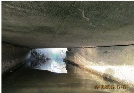
Culvert Barrel; Evidence of Wide Crack and Medium to Severe Erosion
